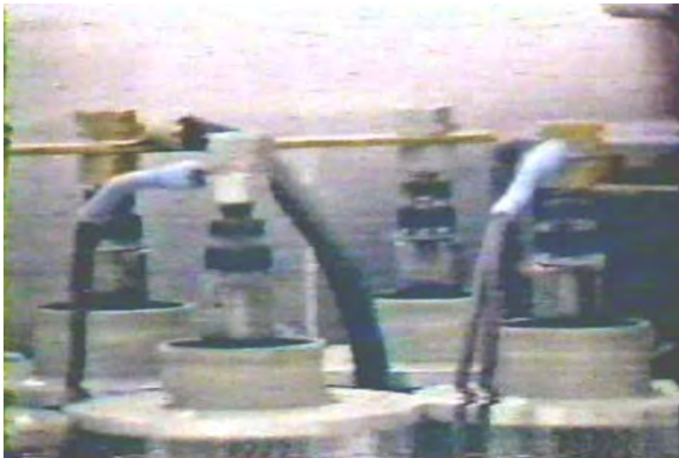
Ignitrons installed on the "Red Motor Cart"
